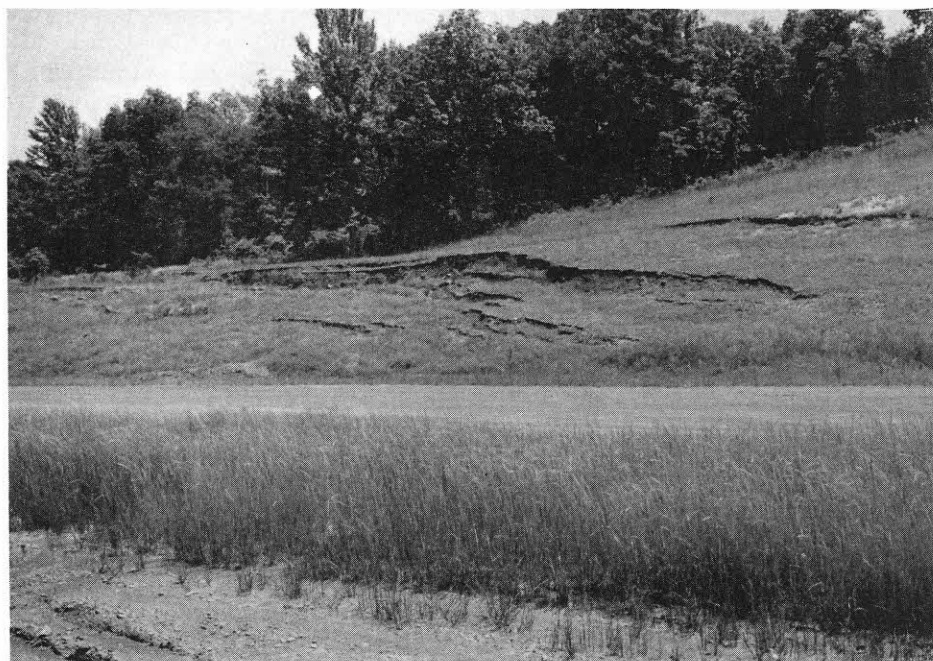
Figure 9 B. -- Minor landslides with a series of crown scarps and small pressure ridges in soils and weathered shales at the northeast part of STOP 2 roadcut.
