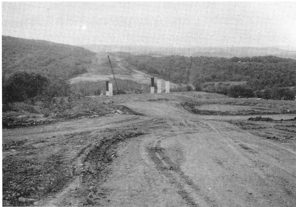
Figure 12 B. -- Excavation, bridge, and buttress walls south of West Fork, Arkansas in lower Atoka and Bloyd strata at STOP 4.
