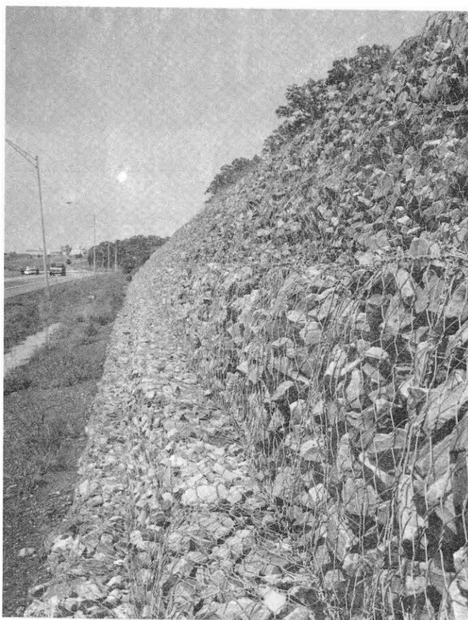
Figure 6 B. -- Closeup showing details of individual rectangular 3-foot meshed wire baskets filled with stacks of rock forming the Gabion wall.
