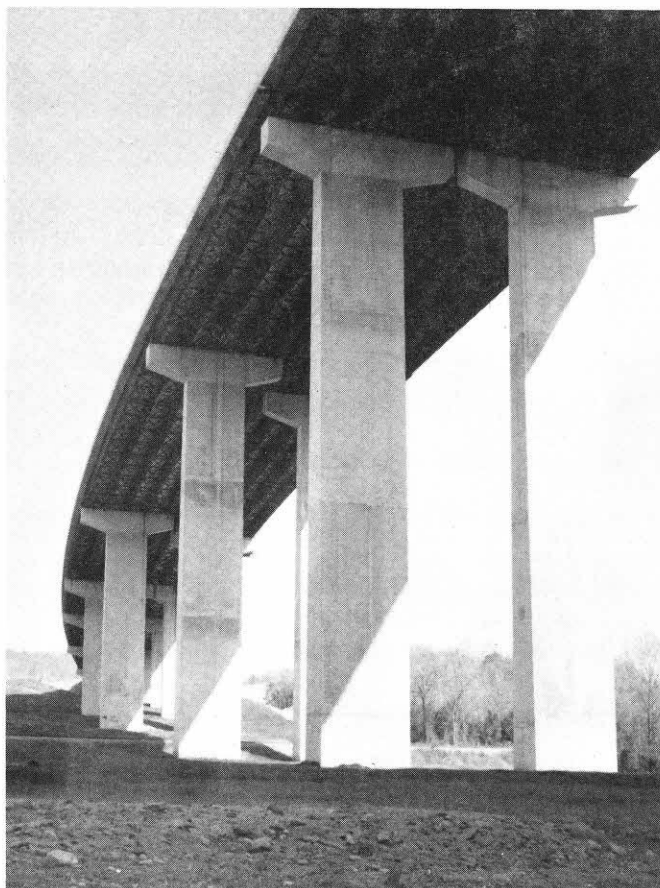
Figure 10 B. -- View of columns and span on 198-foot high and 2287-foot long Frog Bayou bridge.
