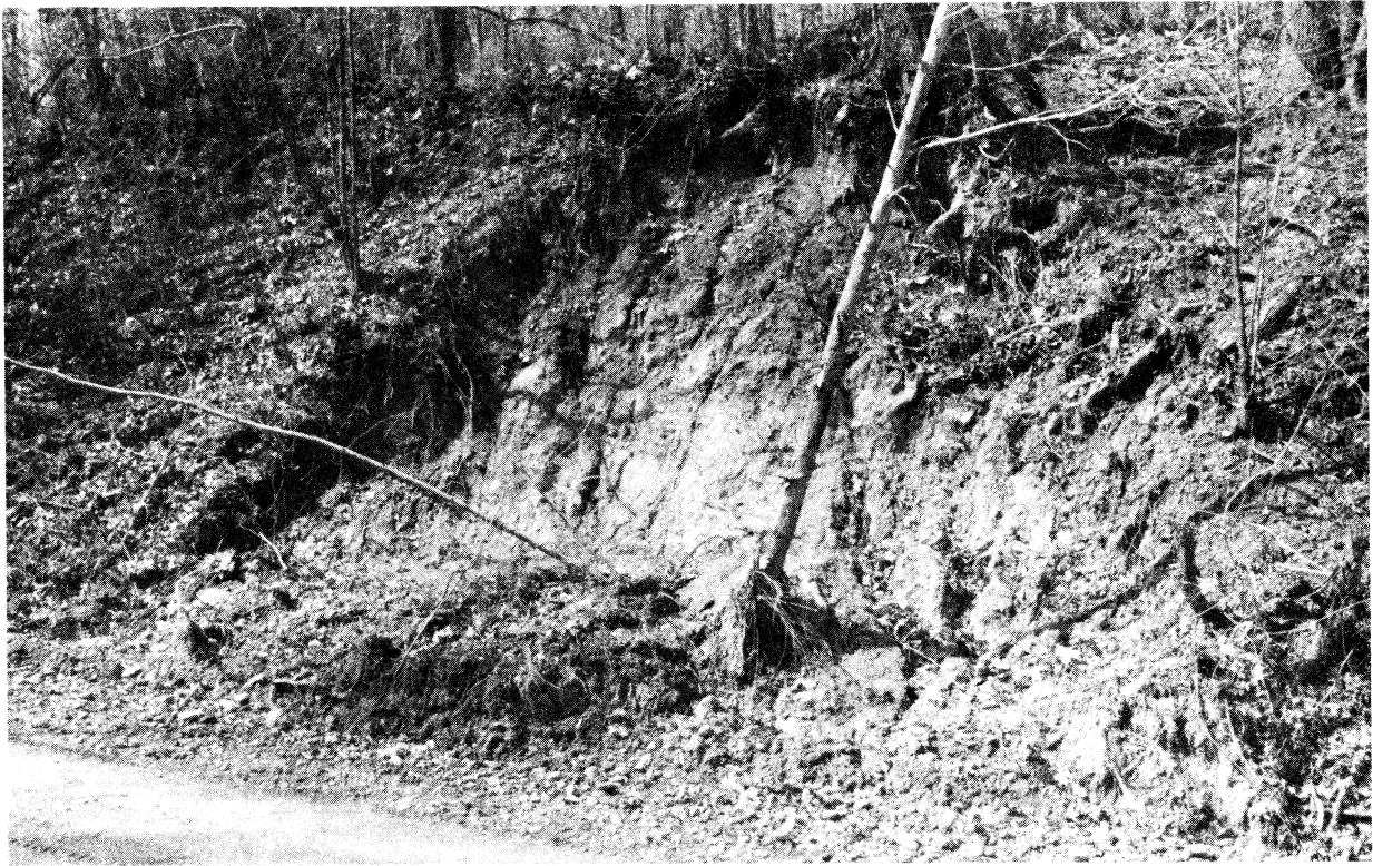
Figure 5. A typical and commonly seen road side rotational slump landslide. Most of the failed debris has been removed by local road crews.
