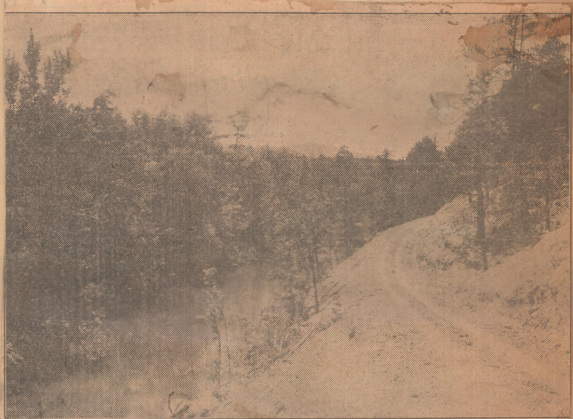
Work being done as a part of the government's five-year development program in the Ouachita National Forest is clearly demonstrated above. This picture, taken along North Fork Creek, shows the Gladstone development road, cut through a heavily wooded section. Such roads as these have been constructed in order that visitors to the forest might penetrate as far as possible into the primitive area.
